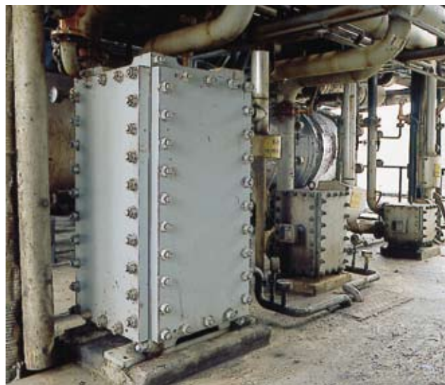
Three Compablocs operating in the atmospheric distillation tower for cooling of kerosene and gas oil.
