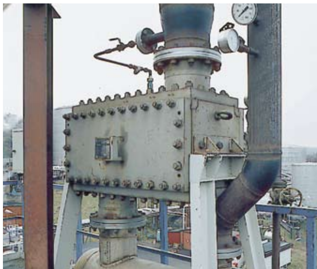
A horizontally mounted Compabloc in titanium used for vapour condensing in the vacuum distillation tower.
